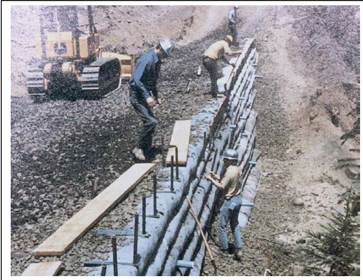
USFS Fabric Wall The U. S. Forest Service built the first ones in the U. S., beginning in the early 70's and produced the first design manual. Co-author of that milestone, John Steward, is in the background.
